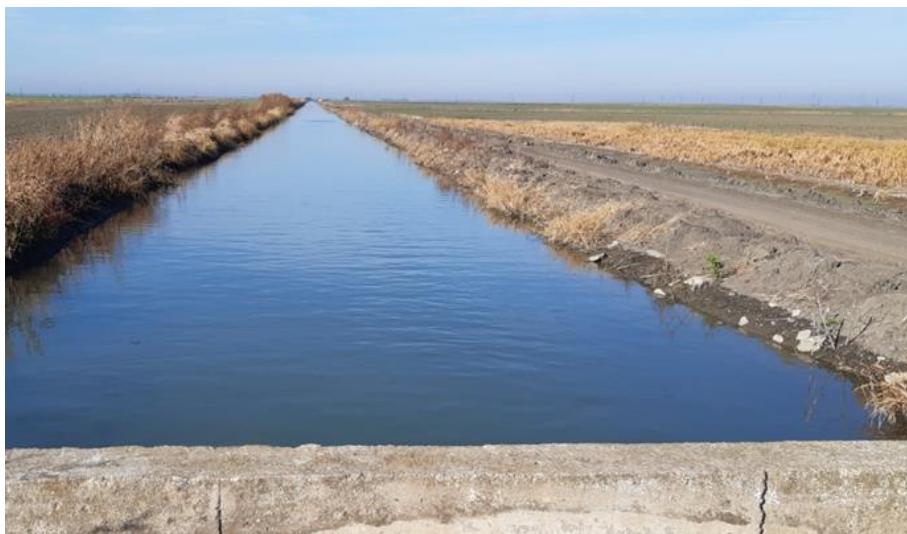
Figura 5.3 Canal principal Figure 5.3 Main channel
