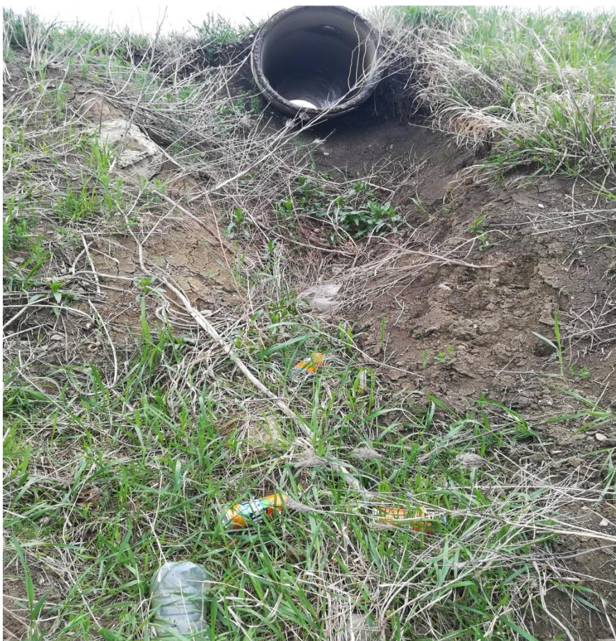
Figura 7.7 Podeț tubular și drum tehnologic agricol degradat (original) Figure 7.7 Tubular footbridge and degraded agricultural technologic road (original)
