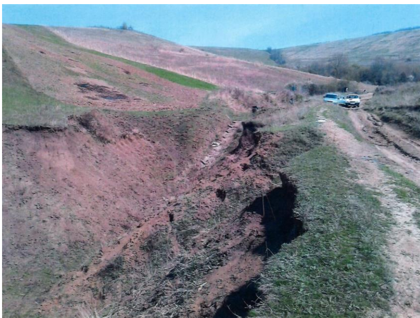
Fig. 4.9 Canal marginal degradat (Oțelești) Fig. 4.9 Degraded marginal channel (Otelesti)
